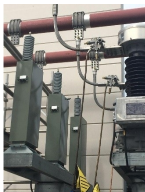
New implemented on site surge capacitor
