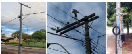
Figure 2 - View of depollution urban centers pole in the synergic electricity distribution and data communications networks at UniverCemig site in Brazil.
