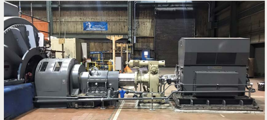
Synchronous Condenser starting using pony motor
