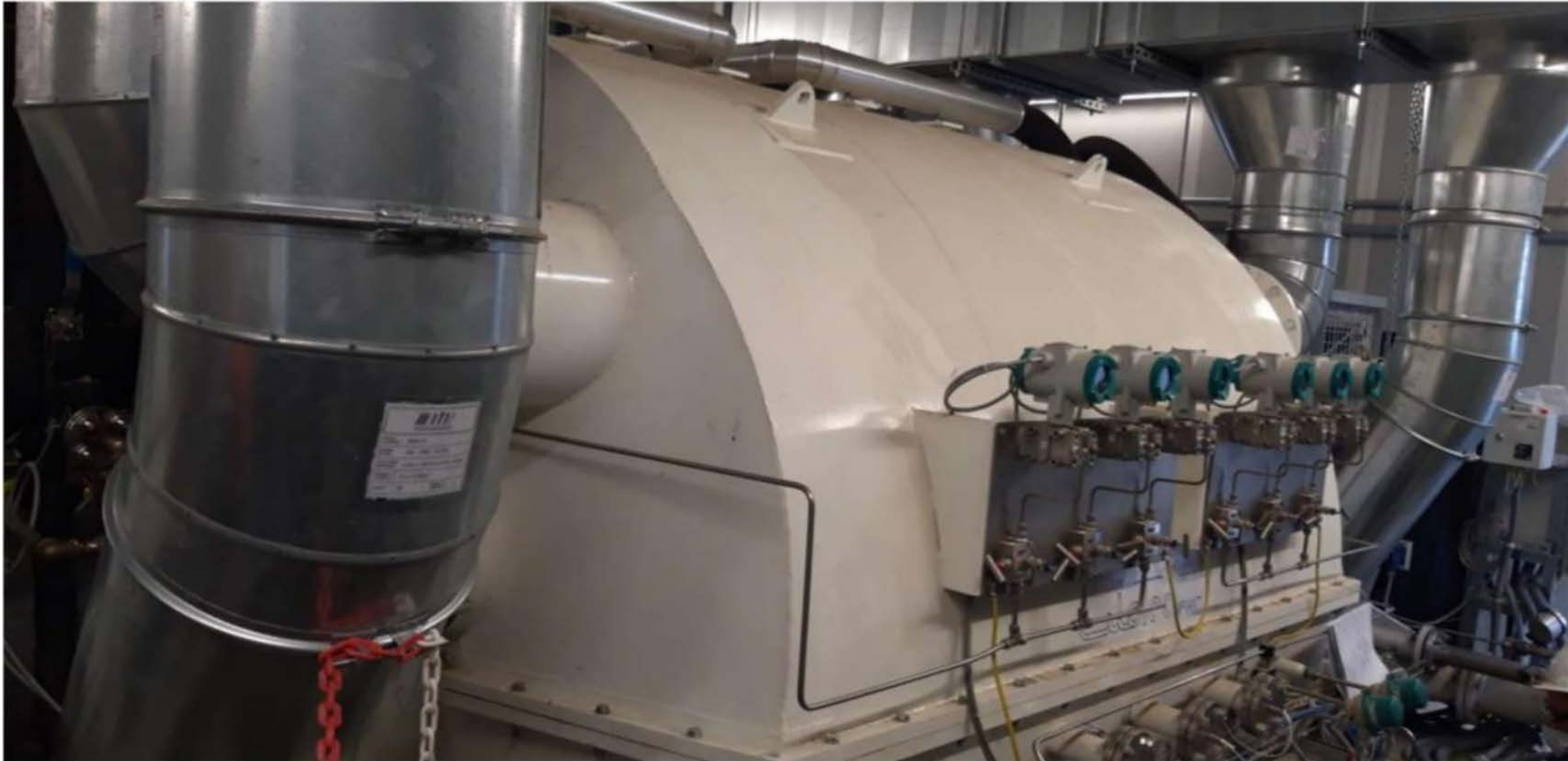
Vacuum tight enclosure for the flywheel (Ansaldo / Criotec).
