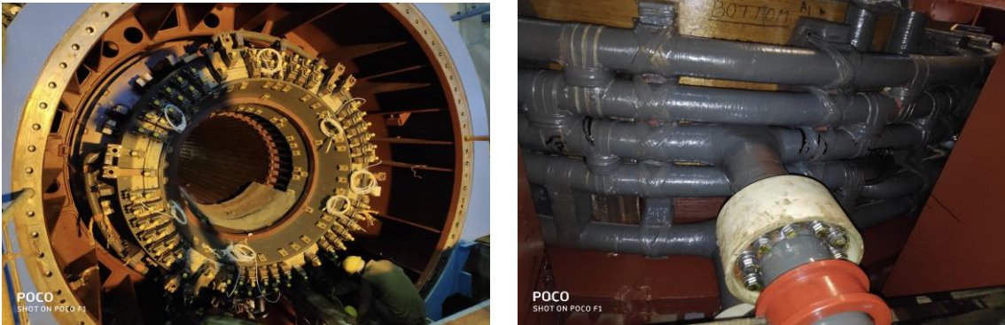
Fig.3a End winding portion of Generator. CBBs can be seen Fig.3b Another view of CBBs
