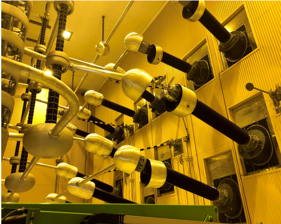
Figure 2. Valve winding bushings of three single-phase transformers
