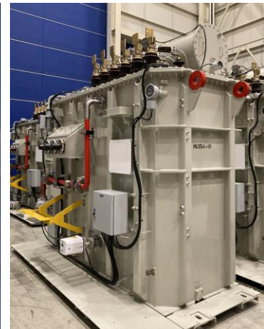
Figure 2 - 14 MVA, 66 kV power transformer
