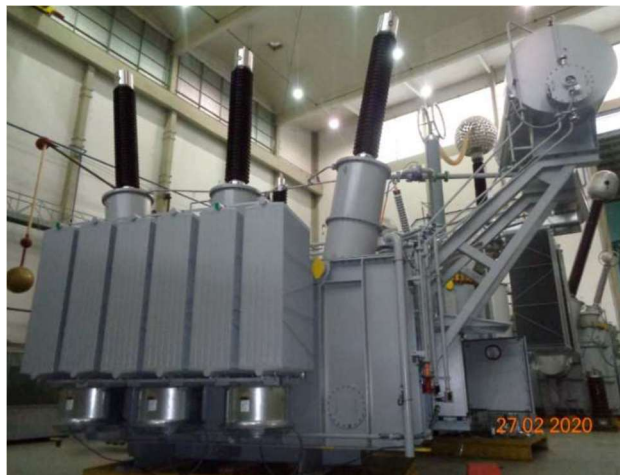
Figure 3 – 200 MVA, 34.5/230 kV natural ester filled GSU transformer – Source: elaborated by the author
