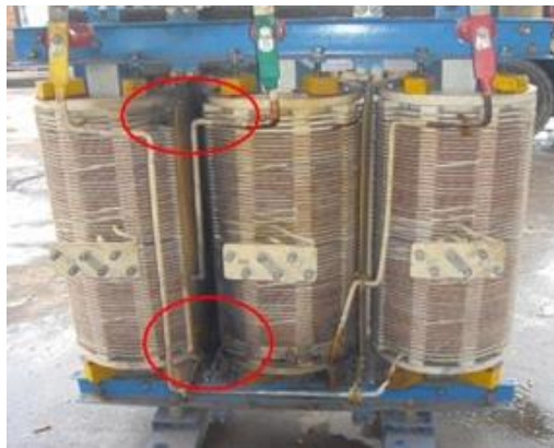
Fig. 2 Photo of partition plate broken down in a 10kV open ventilated dry-type distribution transformer (from the internet)
