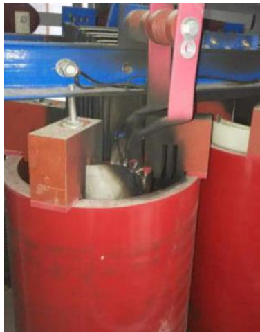
Fig. 1 Insulation broke down between the high and low-voltage winding with a partition in a 35kV cast resin dry-type transformer.
