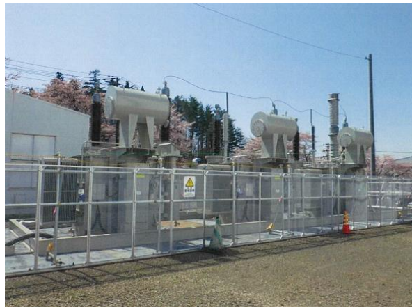
Fig. 6 Appearance during long-term energization test of 3 Units of single-phase, 2 MVA-154 kV model transformer
