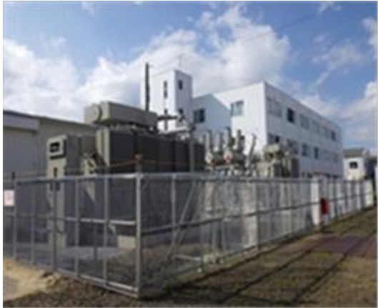
Fig. 5 Appearance during energization test of 2 Units of three-phase, 10 MVA-66 kV transformer
