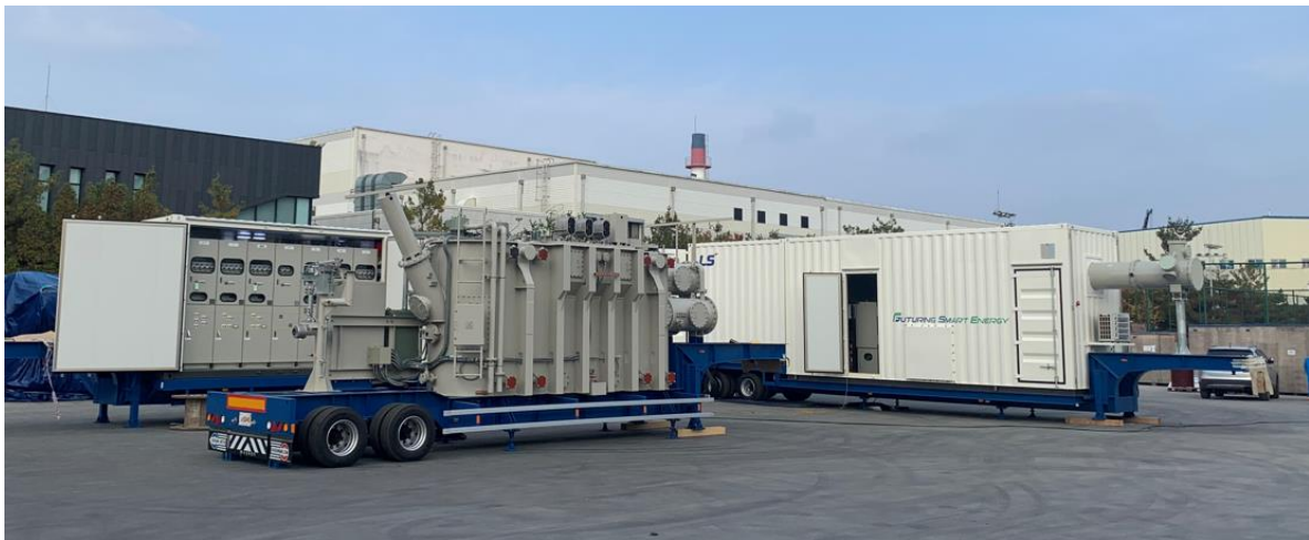
Figure 7 – Interoperation test of modular type equipment
