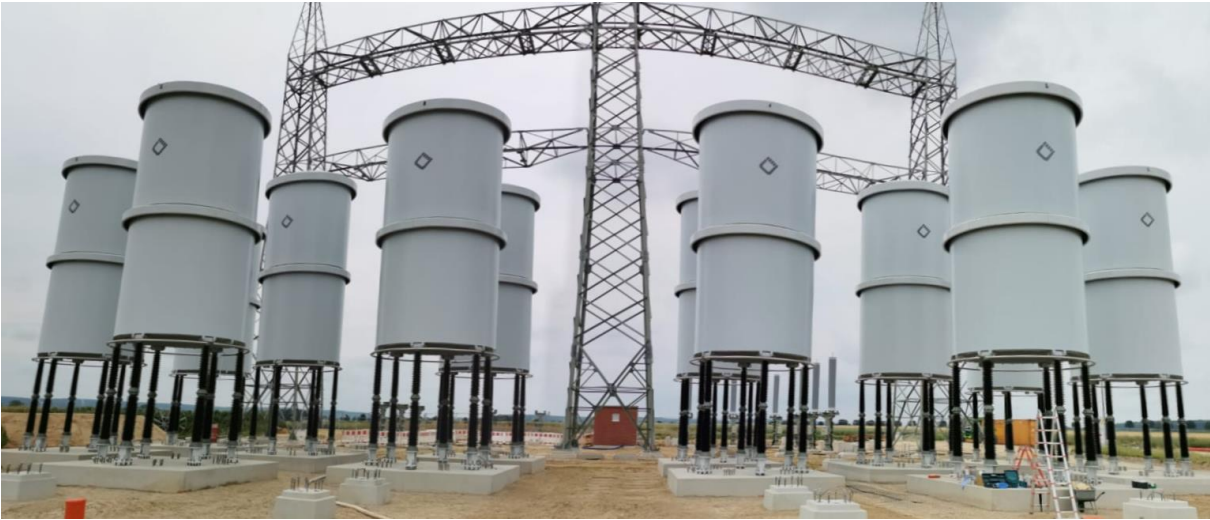
Figure 6: Example of HVSR installation in the 420-kV-system (courtesy of TENNET)
