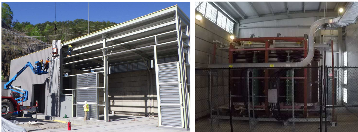
Fig. 8 – The new 145 kV substation: turning the outdoor substation into an indoor one (left); the dry-type 145 kV transformer in service (right)
