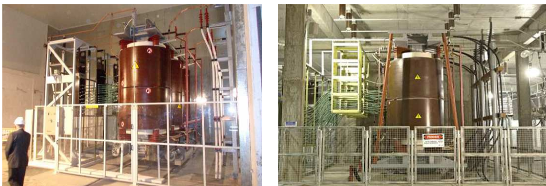
Fig. 2 – Examples of installed 72.5 kV dry-type transformer: four 31.5 MVA units in an urban substation in Spain (left); two 25 MVA in a soccer stadium in Brazil (right)
