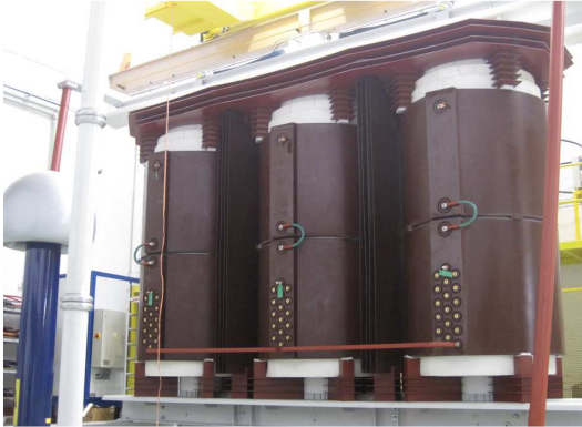
Fig. 4 – 5 MVA demonstrator: main technical data (left); demonstrator being tested (right)
