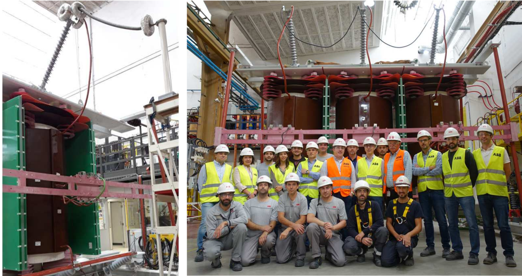
Fig. 7 – The first 145 kV dry-type transformer: testing one phase to validate the design (left); finished transformer after factory acceptance tests with the customers (right)
