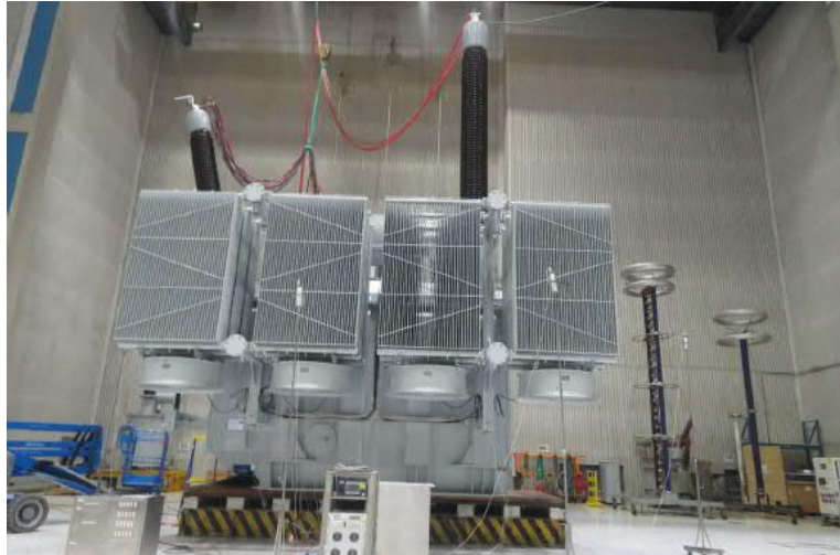
Figure 4 : 334 MVA single-phase auto transformer in the test room
