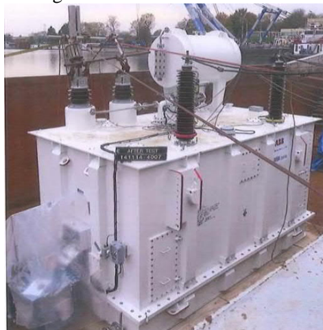
Figure 5. Mock-up transformer of 570 MVA single-phase GSU transformer
