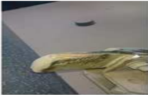
Fig.3.a flashover on earth switch
