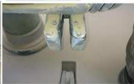
Fig.3.b carbon trace on the earth switch
