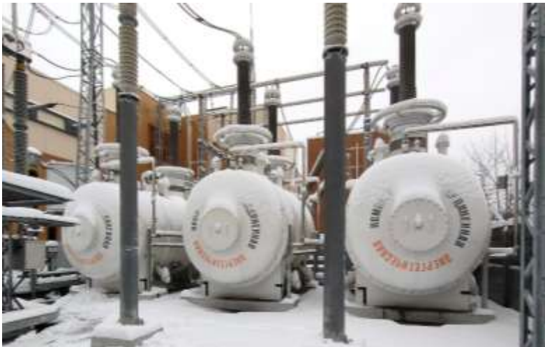
Figure 1 - SFCL 220 kV, "Mnevniki" substation
