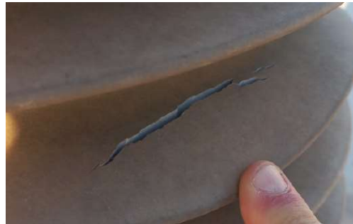
Figure 11: Mechanical damage of shed, most probably caused by shock impact
