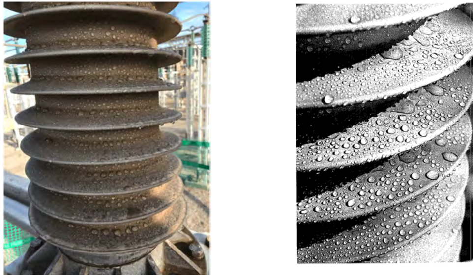
Figure 7: Inspection of hydrophobicity of 72,5 kV hollow core composite insulators, measurement in 2019 (left) vs. measurement in 1996 (right)
