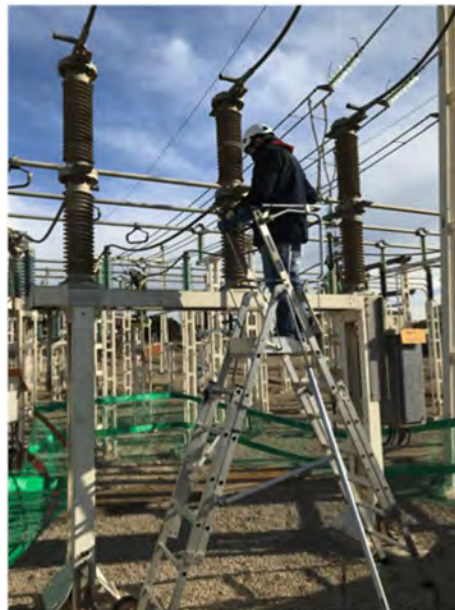
Figure 6: Characterization of pollution level of the insulators by using figure 2 of following IEC/TS 60815-1 (2008) [2]
