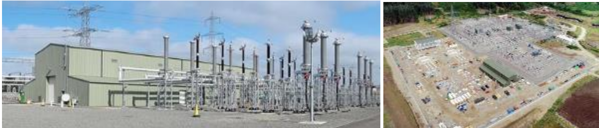
Figure 5-2 – 420 kV substations at New Deer (left) and Fort Augustus (right)
