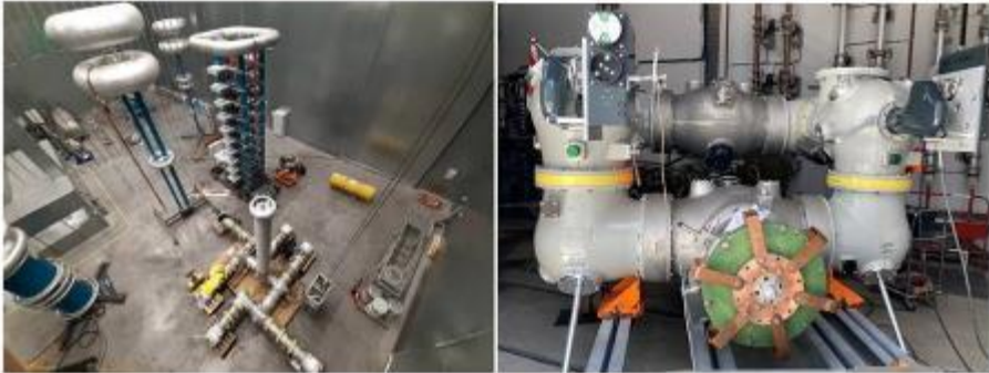
Figure 4-2 – 420 kV GIS devices during dielectric test (left) and bus transfer test (right)
