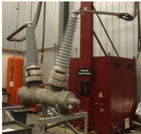
Figure 8 Picture of Dead Tank circuit breaker rated 145 kV under test.
