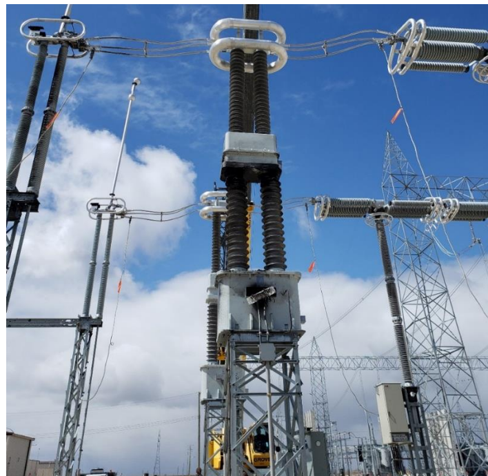
Figure 5 – Riel Converter Station "B" Phase CT After Internal Arcing Fault
