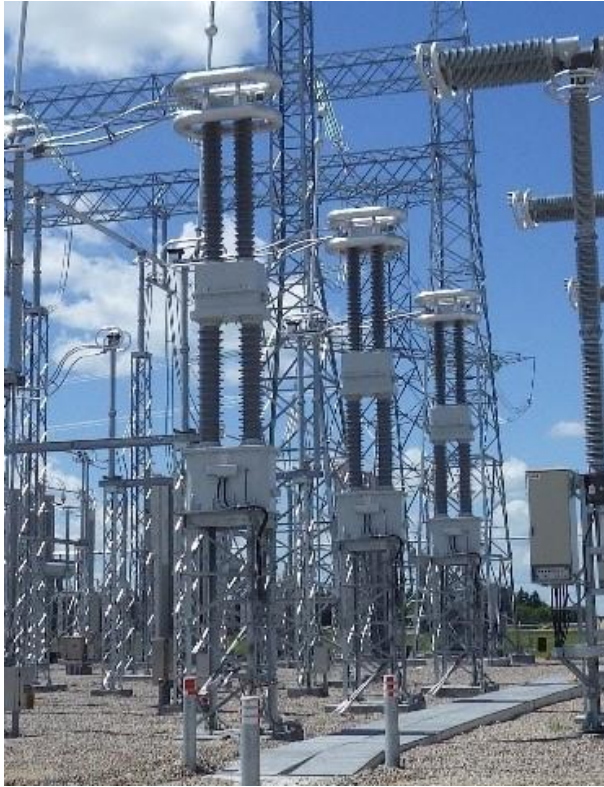
Figure 3 – Dorsey Converter Station
