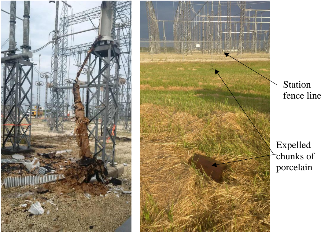
Figure 6 – Dorsey Converter Station 2014 Failure of a 500 kV Oil-Filled CT
