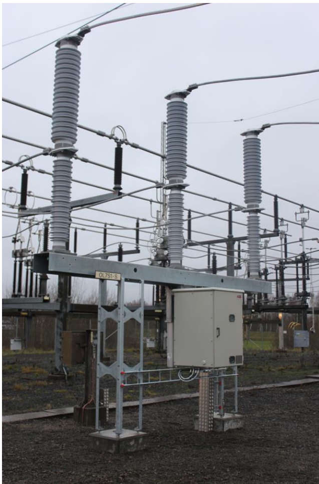
Figure 5. Photograph of the 145 kV, 3150 A (nominal), 40 kA (short-circuit), 50 Hz circuit breaker installed in a substation in Europe.
