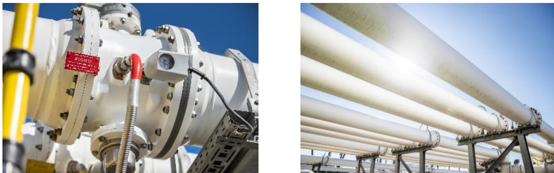
Figure 7: 420 kV GIL at Richborough UK where first Retrofill was performed
