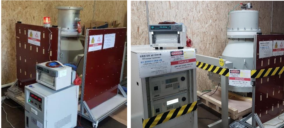
Figure 9. Long term reliability test for single phase (left) and three phase (right) voltage transformer
