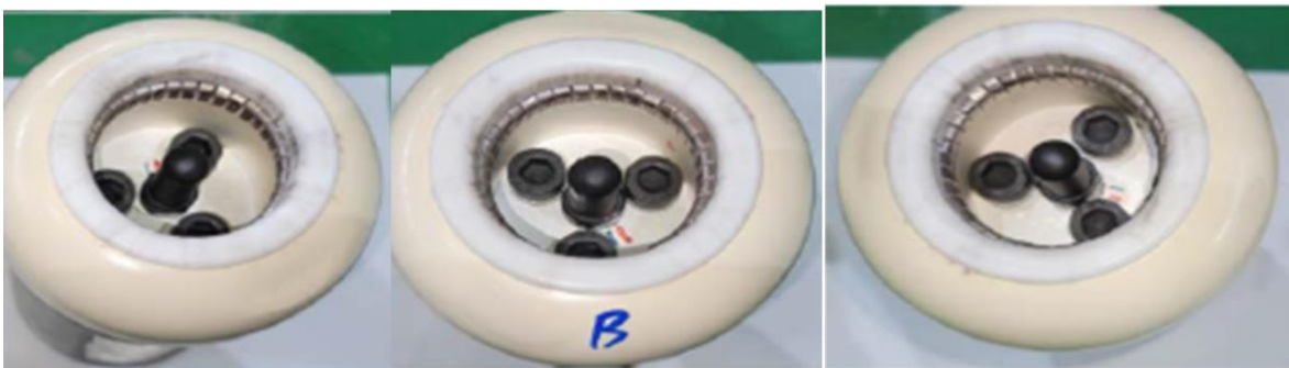
Figure 6. Fixed contact of DS #1 (A phase (left), B phase (middle), C phase (right))
