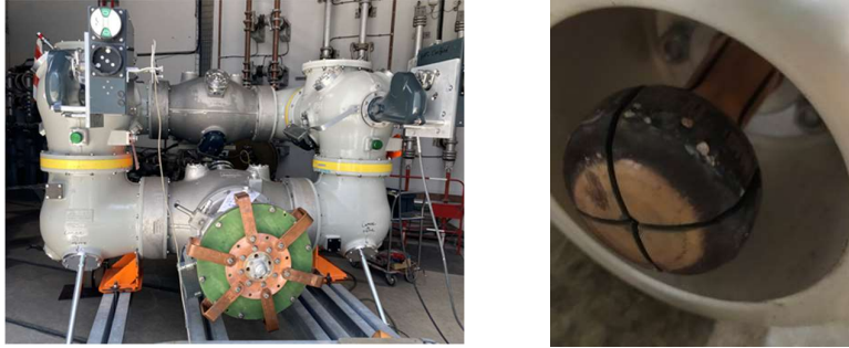
Figure 14: C4-FN/O 2 /CO 2 disconnector in bus transfer current switching test (left) – arcing contact after test (right)
