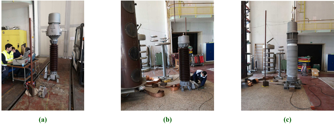
Figure 2 Transformers considered in this paper. (a) CT Type AGU-123 (b) VT Type VPU-123 (c) SSVT Type VPT-145 50 kVA
