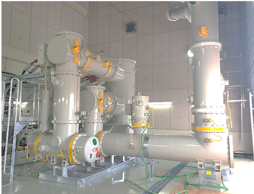
Figure 10. Complete GIS in operation in the Wanggok substation in South Korea
