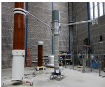
Figure 4: 245 kV combined transformer during type tests
