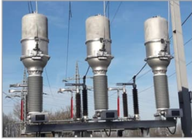
Figure 6: First pilot installation of 123kV synthetic air combi in German substation [12]
