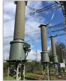
Figure 7: 420kV synthetic air voltage transformer installed in German's TSO grid.
