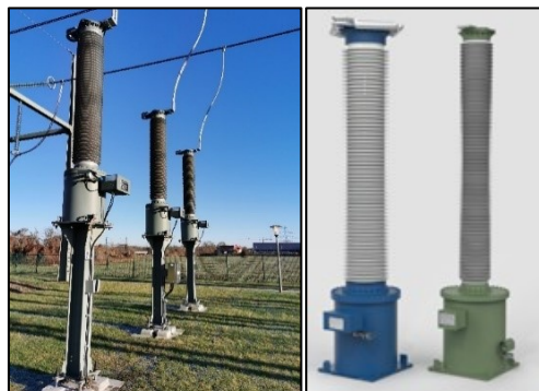
Figure 7: Left: 245 kV Clean Air VT at substation Wambel (source Amprion); Right: Comparison of Clean Air (blue) und SF 6 (green) 420 kV VT
