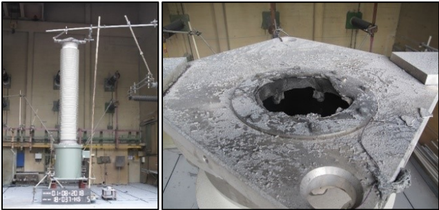
Figure 2: 420 kV VT after internal arc fault test with 80 kA and properly triggered rupture disk.
