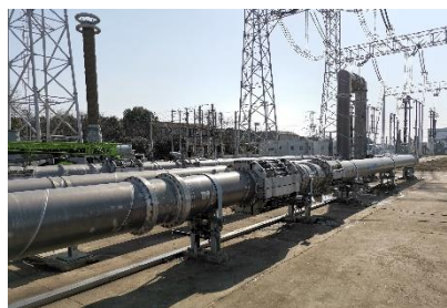
Figure 7 Live test of 1000 kV environmental GIL prototype at UHV AC test base.
