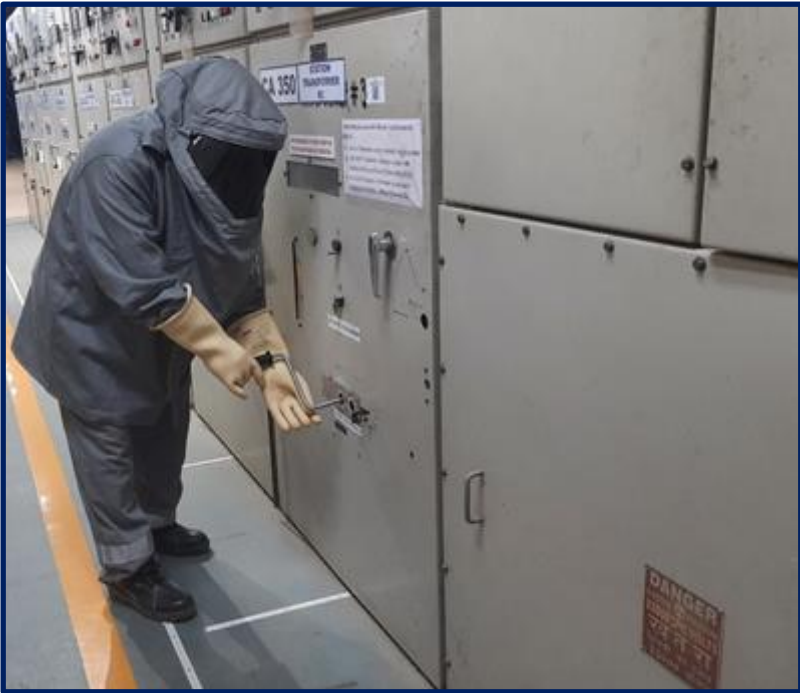
Figure-2: Operating person wearing Arc suit for carrying out rack in & rack out of breaker
