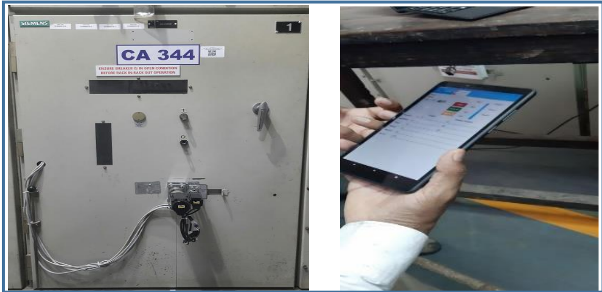
Figure-6: Motors mounted on the breaker panel & Mobile app
