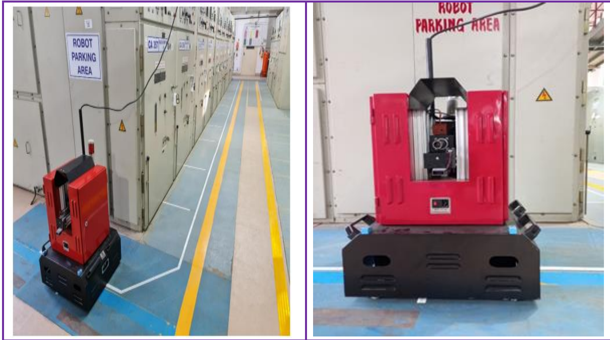
Figure-10: Robot images in switchgear room
