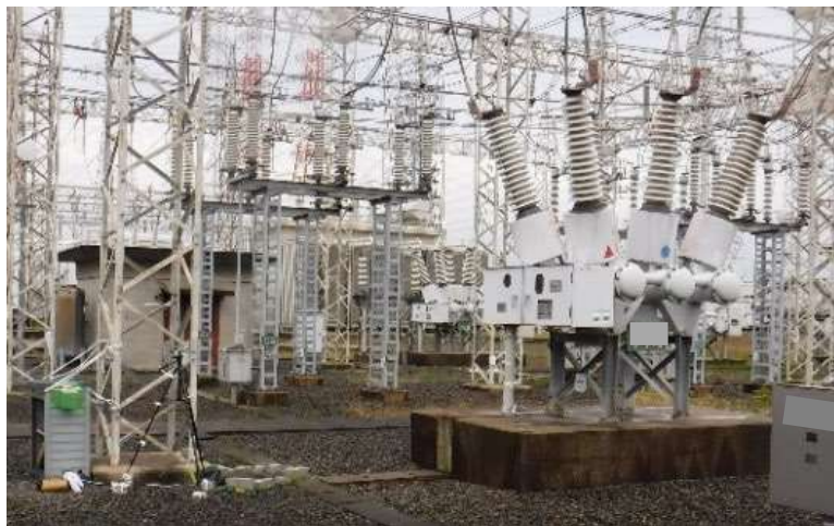
(2) Trial situation at the actual substation
