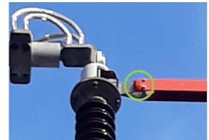
Figure 7 Temperature sensor integration in the main contact
