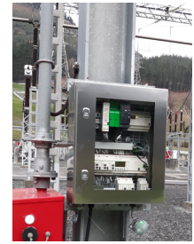
Figure 6 Controlbox integrating all the IED's for the ADCM disconnector
