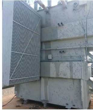
Figure 6: 138 kV to 69 kV Autotransformer Oil Leak [4]
