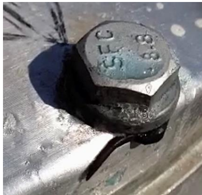
Figure 9: Bubbling due to SF 6 Leak on 345 kV Circuit Breaker
