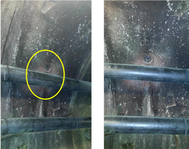
Figure 4: Example of a 400kV Cable fault in a Tunnel Installation (20 kA rms fault current / 80ms fault duration; I x t = 1.60 x 10 3 )
