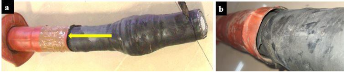
Figure 2: Images near the cable junction: a) the heat shrink tube slipped away from junction highlighted by yellow arrow and b) gap visible between heat shrink tube and internal layer of termination
