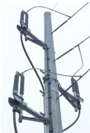
Figure 10: Dry terminations with surge arrester on tower
