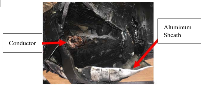
Fig. 6 Status of insulation breakdown (magnified)
