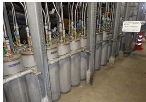
Fig. 24 Disaster prevention equipment for TJ (fire extinguishing system)
