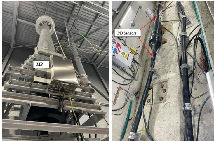
Figure 10: a) Monitoring Point under the DC outdoor termination b) PD sensors placed on the HV joints
