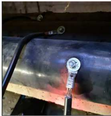
Grounding device to connect the core and the screen of the cable
