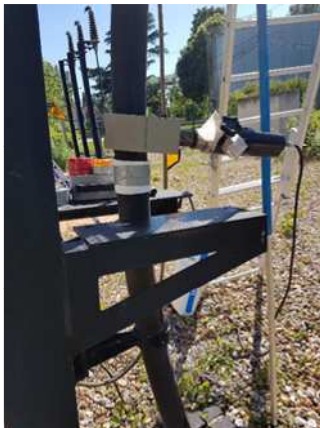
Absence of voltage check under a cable sealing end
