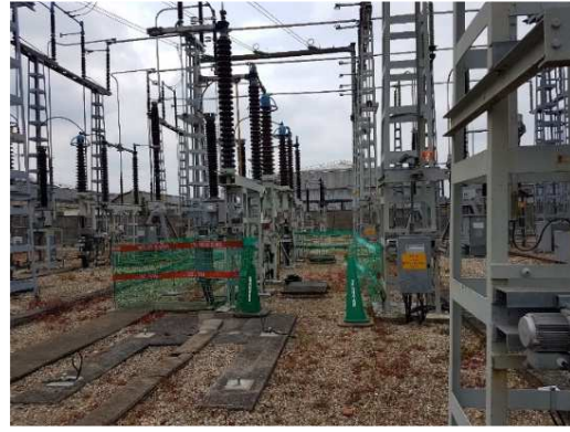
Connections in the RTE substation to the other side of the High voltage link
