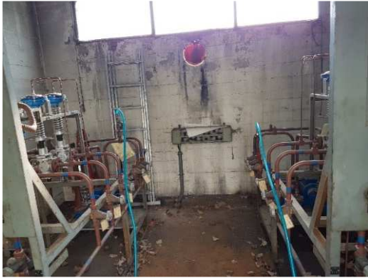
Connections in the fluid station of units 3 and 4 in the power plant
