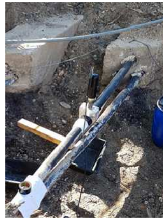
Absence of voltage check in excavation to safety cut the cables
