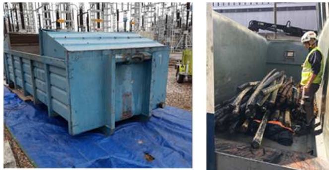
Watertight container with a roof to store cables
