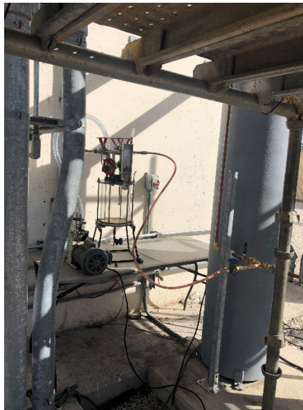
Fig. 12: Vacuum Treatment Setup
