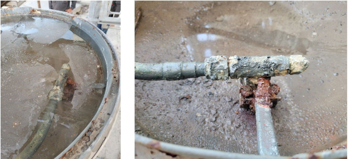
Fig. 5 and Fig. 6: Corroded Oil Reservoir Valves and Fittings
