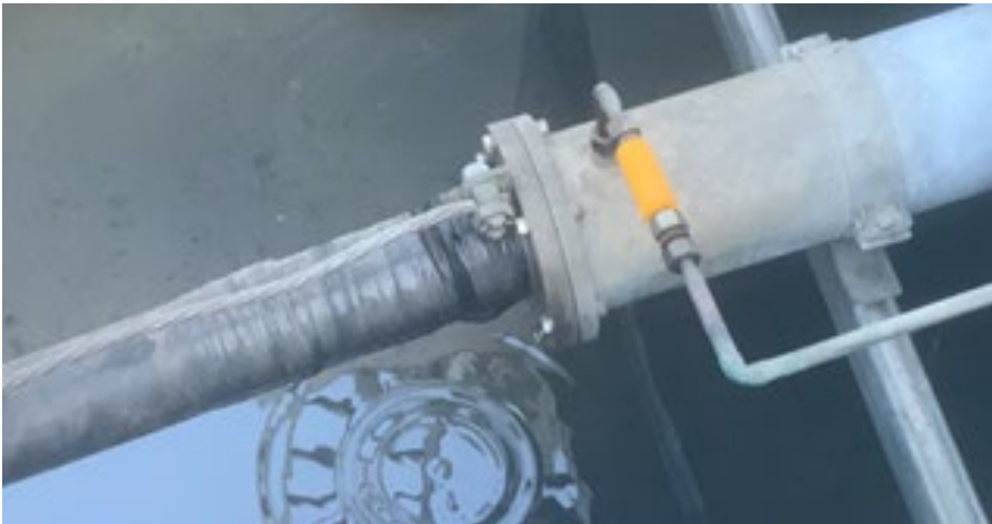
Fig. 4: Leak Sealed with Plastic Cling Wrap and Tape
