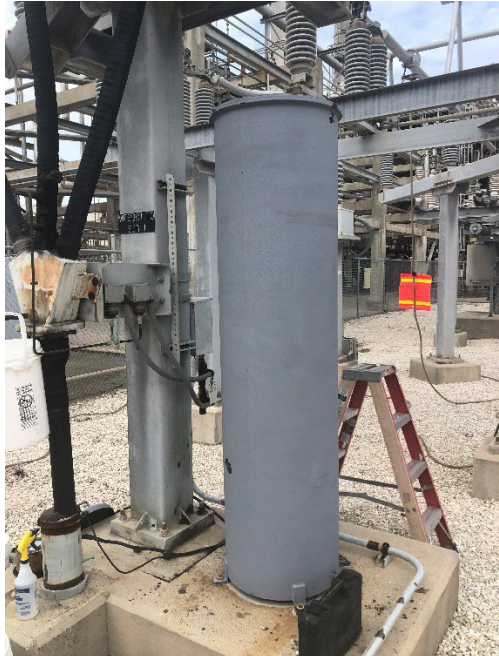
Fig. 8: New Oil Reservoir – Outdoor End
