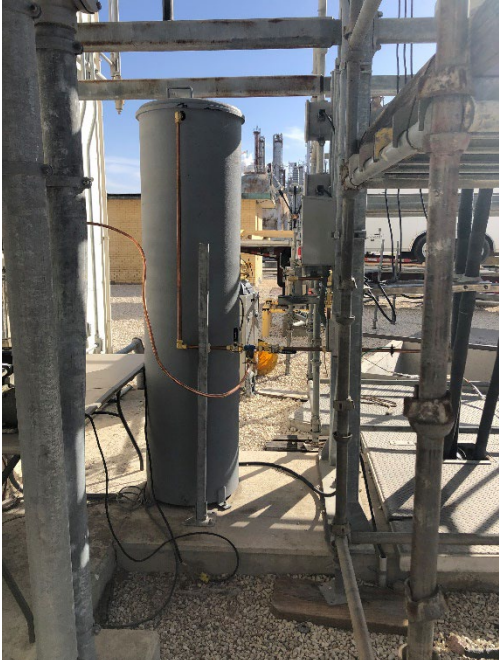
Fig. 7: New Oil Reservoir – Substation End
