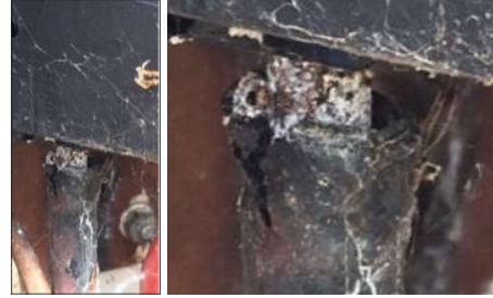
Figure 13 – example of charred cable insulation and high temperature corrosion
