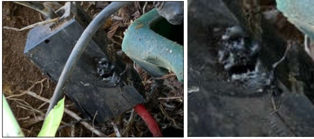
Figure 12 – example of heat damage to a black fuse carriage and the indentation on the green pillar mounting plate
