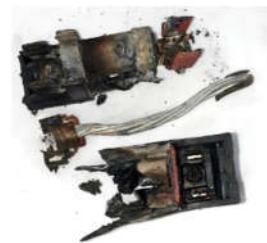
Figure 10 - Example of a failed fuse and fuse holder
