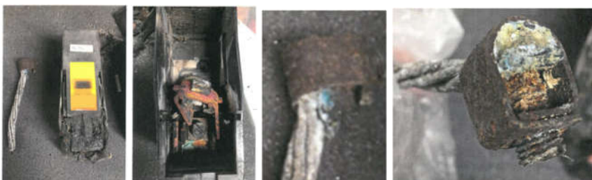
Figure 11 – example of aluminium cable conductor of which the insulation has charred off (left), the heat damaged fuse holder base and insert (right) note the grub screw and part of the connection plate still connected to the conductor.
