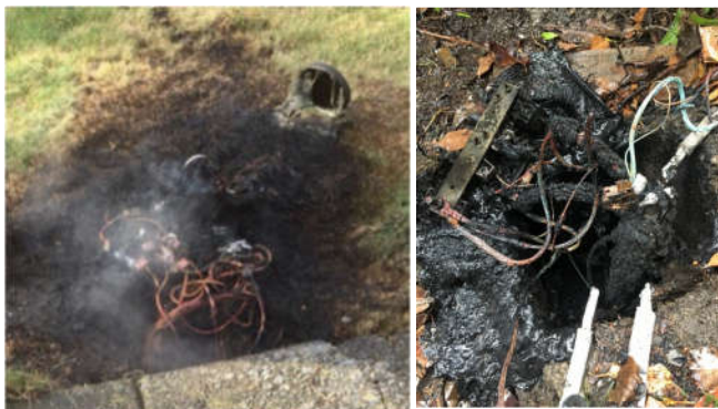
Figure 2 – the remains of two other plastic pillars after a fire
