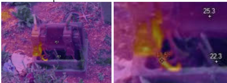
Figure 15 – Hotspot at the Bottom of a Fuse Holder: bottom end of the fuse holder at 48.5°C, mounting plate at 25.3°C, incoming cables at 22.3°C
