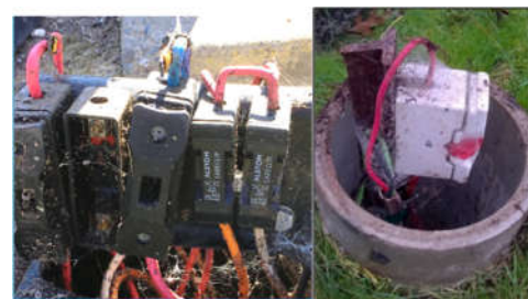
Figure 3 – examples of internal LV pillar components: mainly fuses, relays and links
