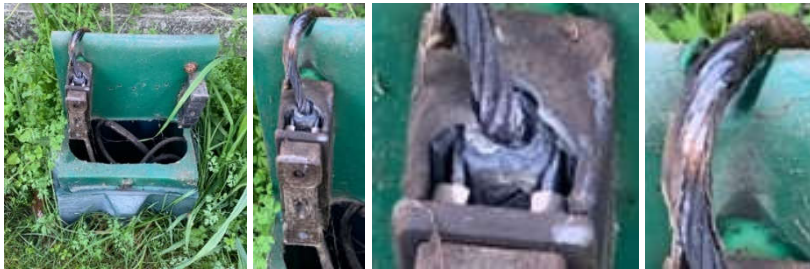
Figure 14 – example of heat damage on the fuse holder and cable as charring, and the disappearance of cable insulation above the fuse holder. damage to the plastic body as whitening of the plastic above the fuse holder, charring of the plastic above the fuse holder, and an indentation of the cable in the top of plastic back plate
