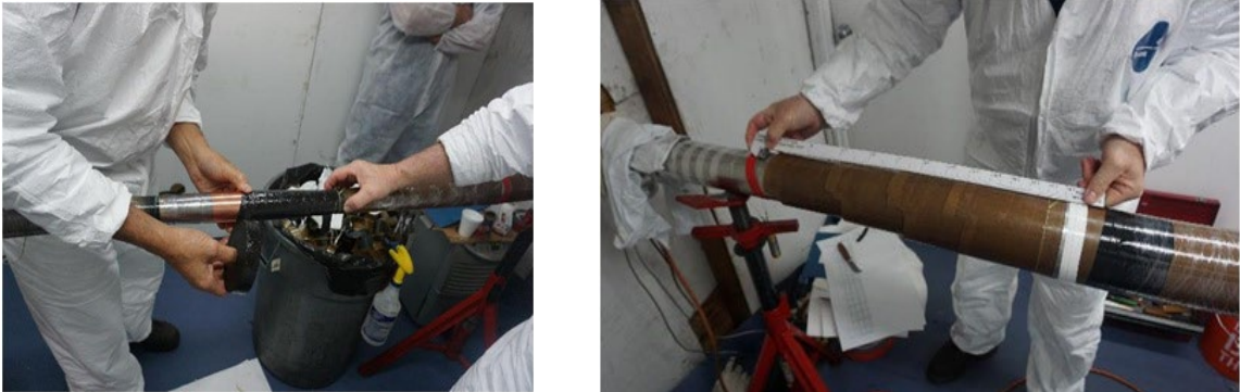
Figure 3 : Installation of 345 kV LPP joint – shielding of the connector (left), template for the stress cone slope (right)
