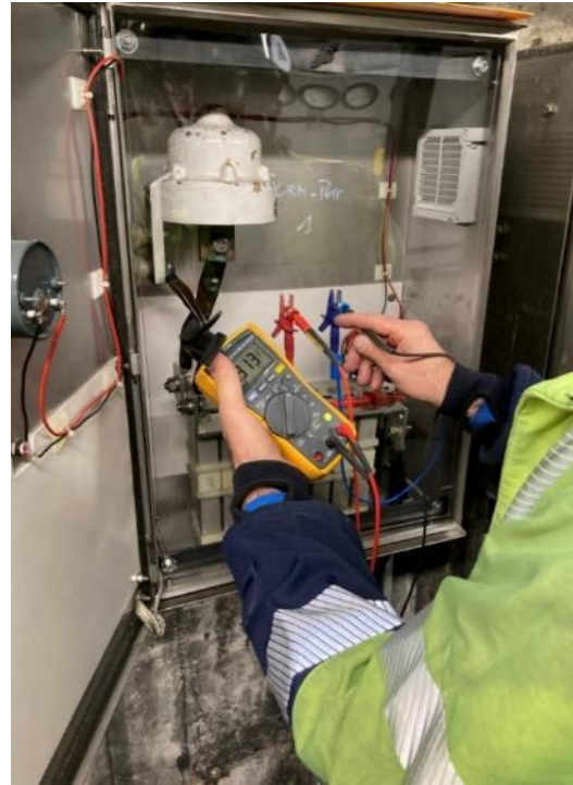
Figure 7: Monthly maintenance visit of a battery ensuring cathodic protection
