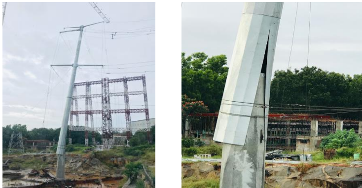
Fig 24. Failure of shaft.
