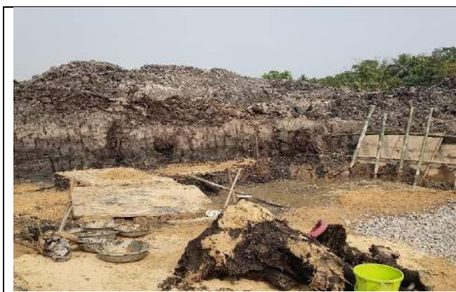
Exhibit-2: Decomposed soil with water logging
