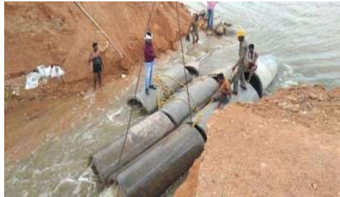
Figure 4: Photograph of approach road washed away due to flash flood
