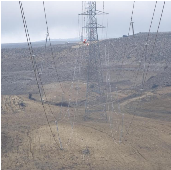
Fig.3 – IPS on a 154kV DC line
