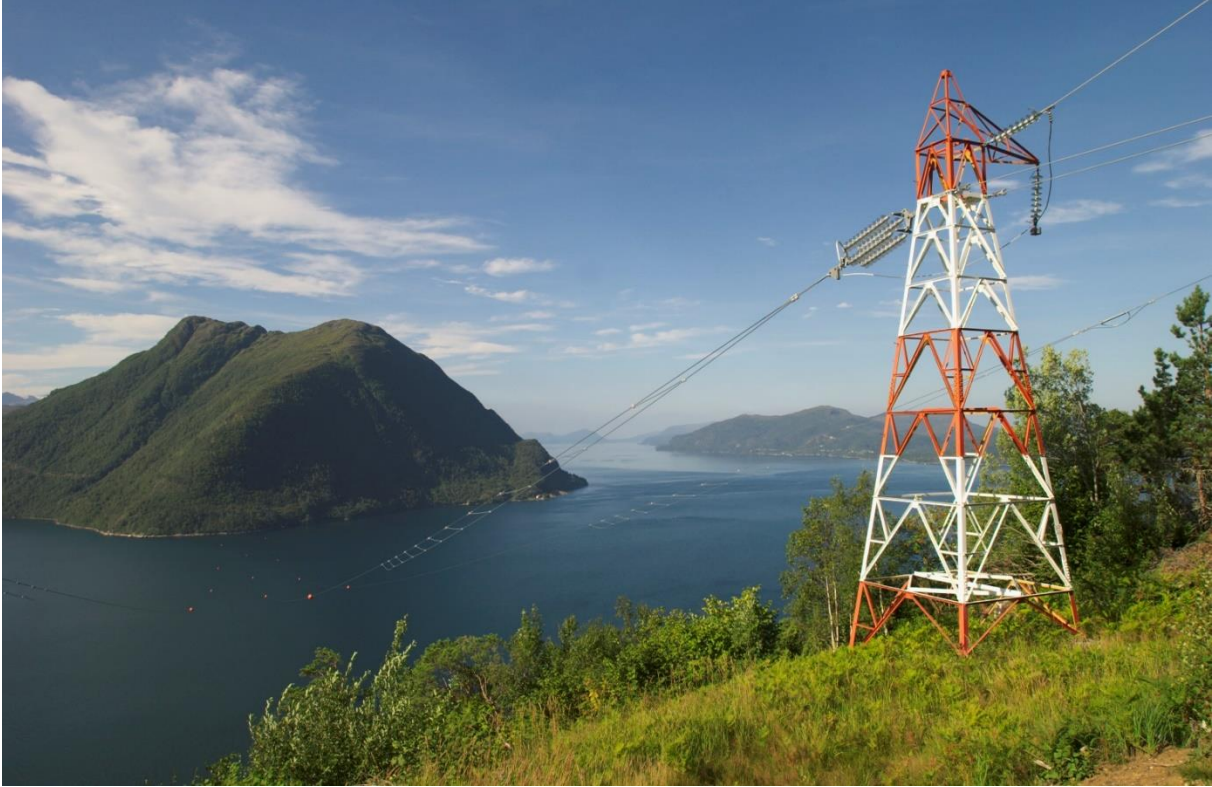
Figure 2 - Former Stor fjorden crossing with an older tower type and a damper loop arrangement
