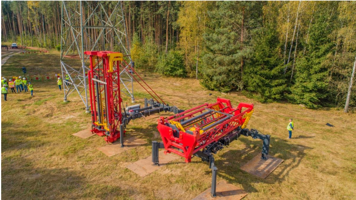
Figure 9. Tower after installation of extension, Device in both position operational and transporting.
