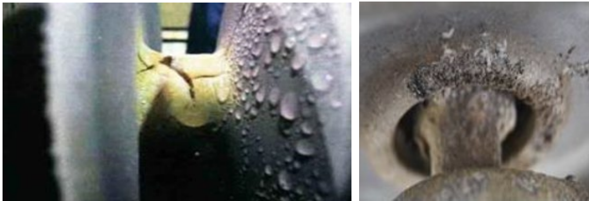
Figure 2 (Left): Erosion of a polymer insulator which is still hydrophobic after approximately 15 years in service in harsh conditions. (Right): Comparative erosion of a silicone coated glass insulator.
