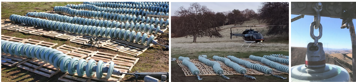
Figure 7: Example of under coated glass insulators installation at PG&E
