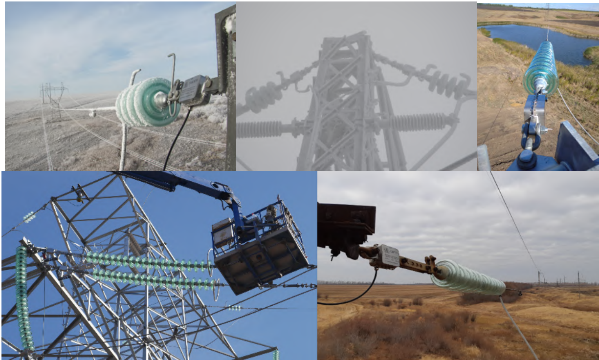
Figure 4 – FBG load-cells installed on Overhead Lines
